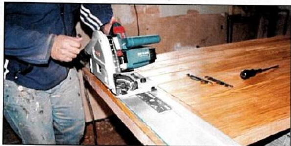
Although ideal for converting sheets, it's perfect for door fitting as well
